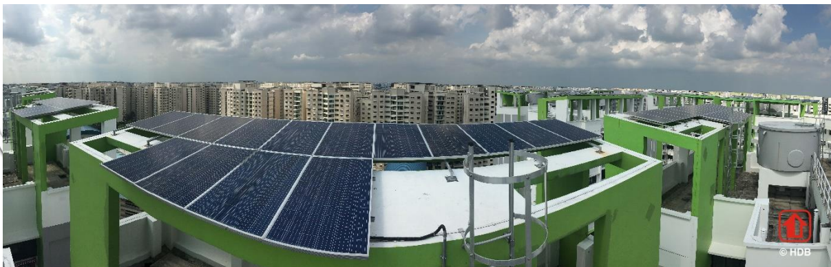
The solar-ready roofs piloted at Punggol Edge BTO project were inbuilt with infrastructure to enable seamless installation of solar panels to harness renewable energy for block services
