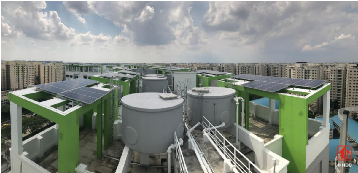
Essential block services such as water tanks and lift motor rooms were strategically located to optimise available space for installation of solar panels on the roofs, with access routes planned for easy maintenance
