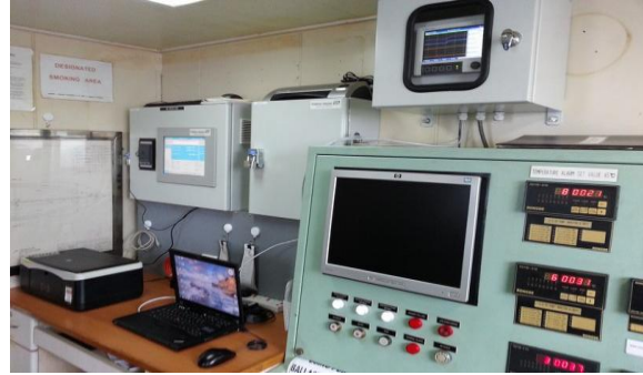
Endress+Hauser's Bunker Metering Computer
